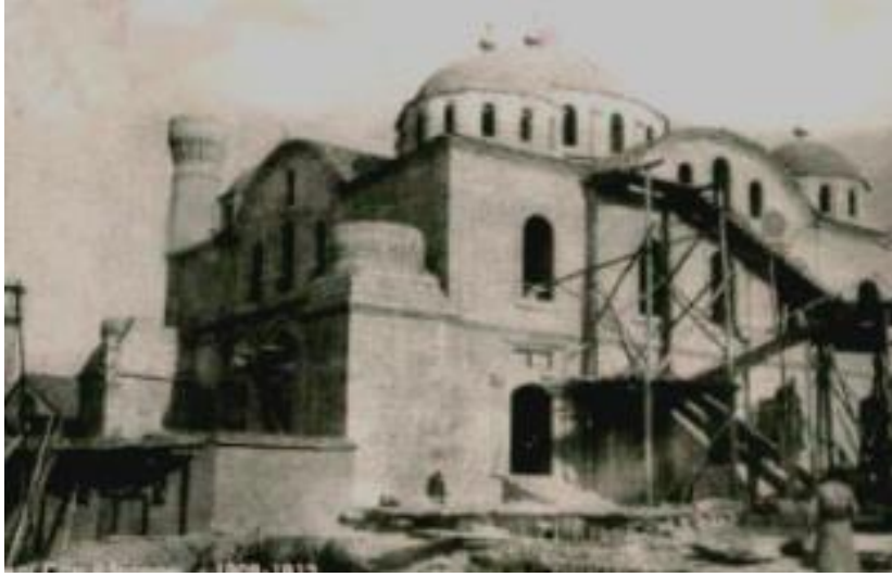
Figure 3. Damage and restoration of Malatya Teze Mosque after the 1964 earthquake [29]
